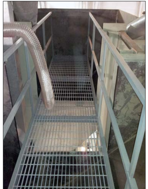
Catwalk installed over the large seed hopper allows for easy access, facilitating the loading and stirring of seed.
