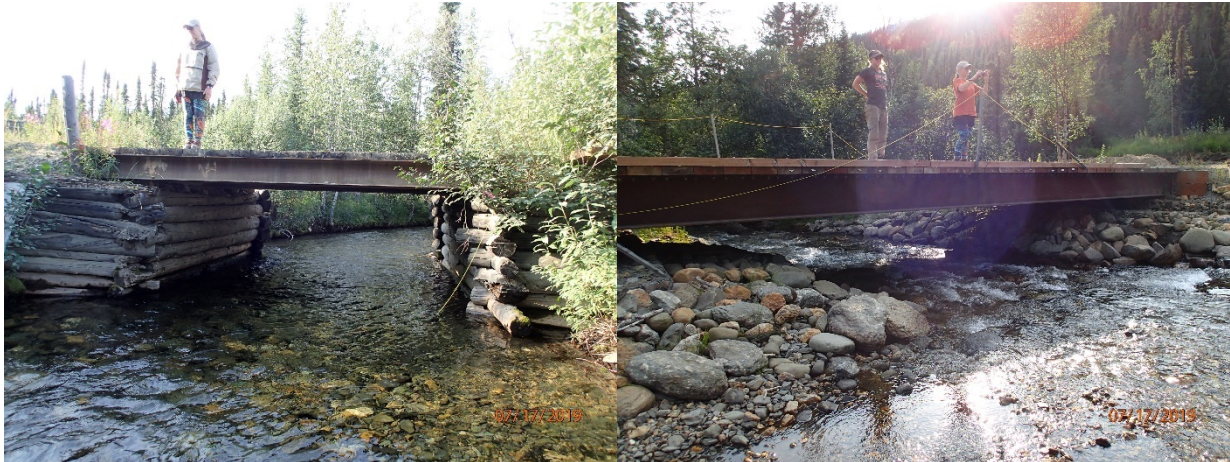
Figure 13. Bridges over Dahl Creek (left) and Wesley Creek (right) in July 2019. The Dahl Creek bridge is scheduled to be replaced in 2020.
