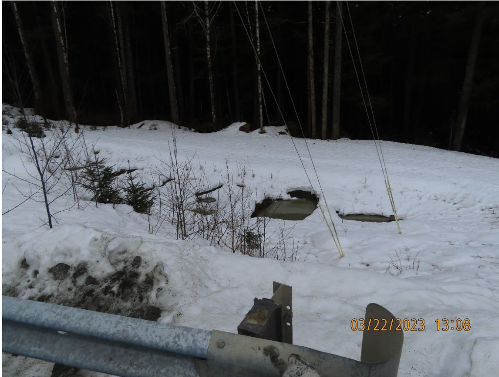
Photo 10. "Gnome Pond" stormwater ponds.
