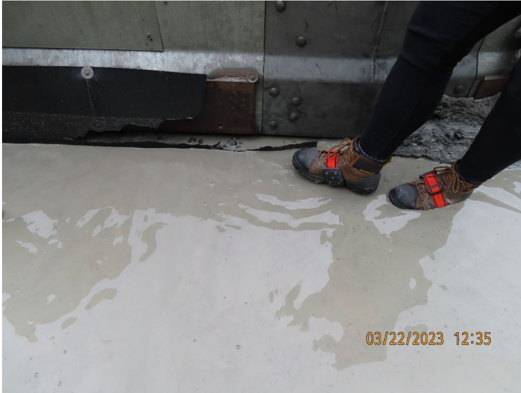
Photo 6. Killer Creek Bridge liner damaged, allowing turbid water to infiltrate.
