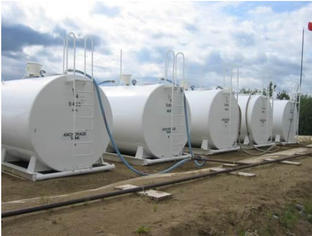
Figure 21: Fuel Storage Site
