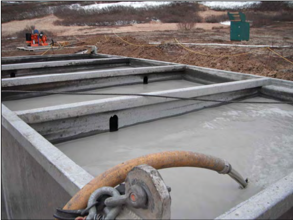
Figure 2. Recirculation tank in use. Drill water from final sump pit is recirculated back to drill for reuse.
