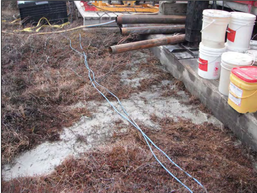
Figure 13. Presence of drill water on tundra adjacent to storage location of additives. This appeared to be overflow from the trench between drill hole and sump pits.
