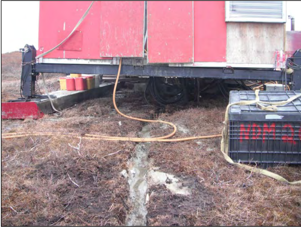
Figure 11. Trench transferring drill water from drill hole to the series of sump pits for settling out and recirculation.
