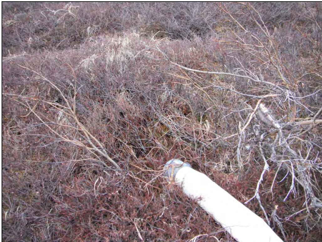
Figure 14. End of sump pit discharge line. Because drilling was shut down, no discharge was occurring during the inspection.
