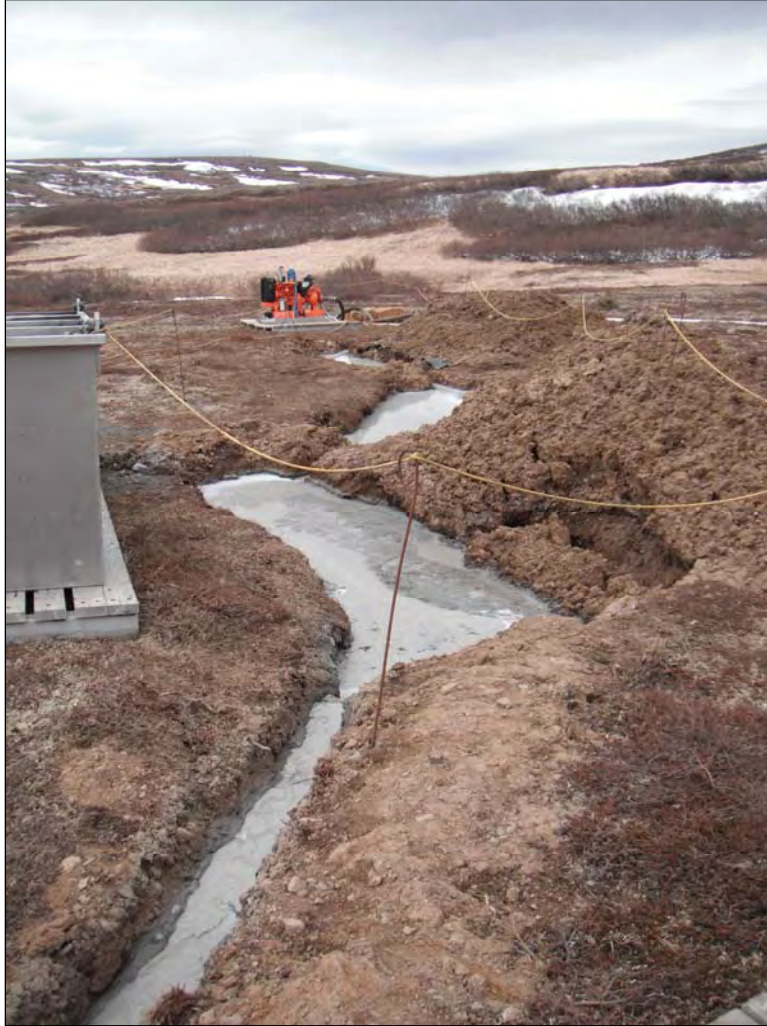
Figure 3. Series of sump pits (left) and stockpiled muck (on right) to be used later in site reclamation.
