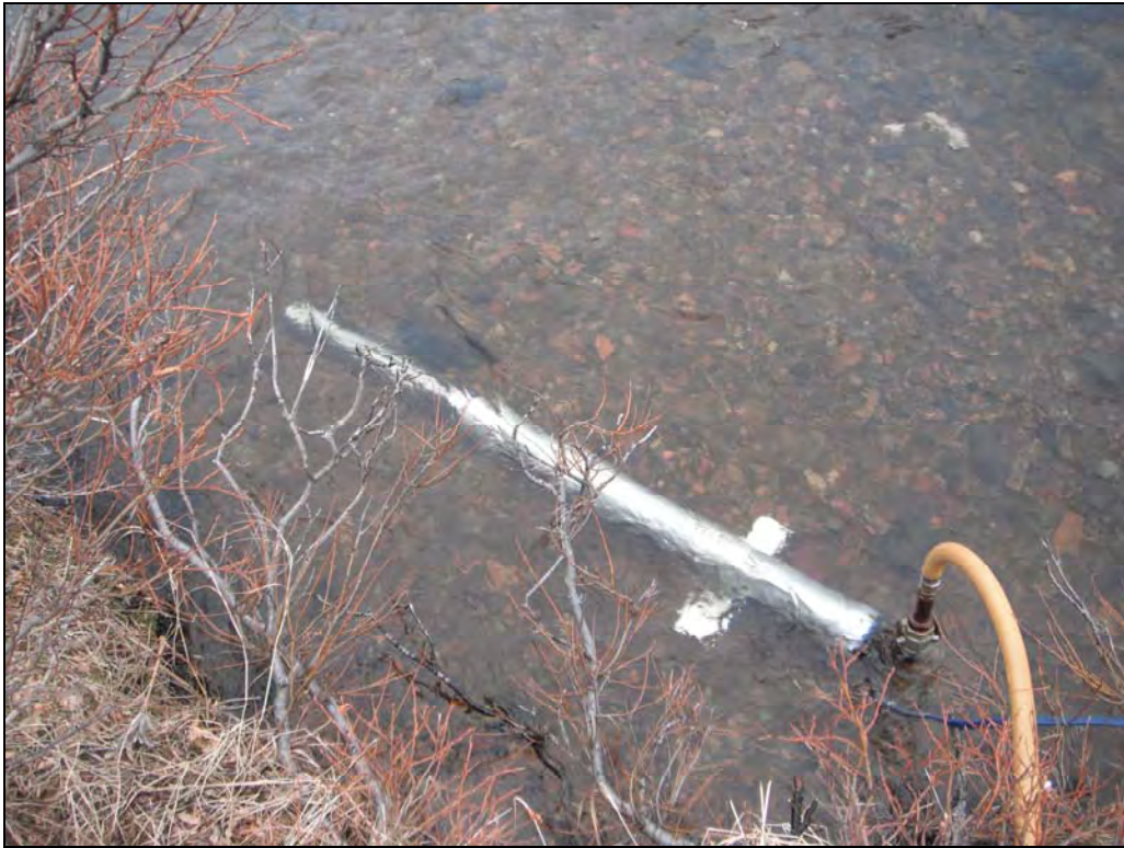
Figure 17. Screened water intake submerged in creek.
