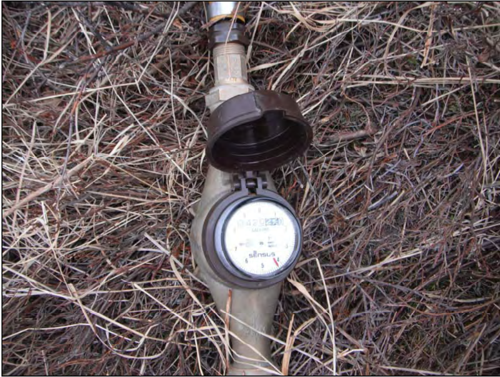
Figure 9. Totalizer connected to water intake line. Field estimate of water withdrawal rate was 23 gpm during the inspection.
