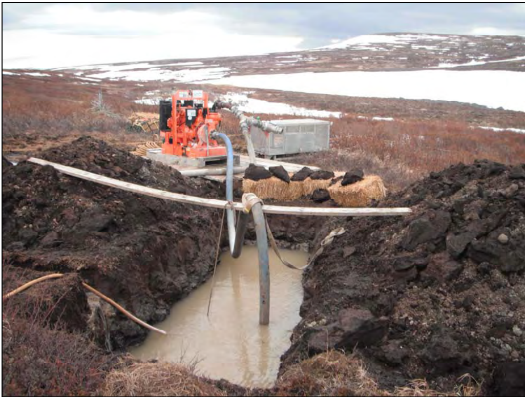
Figure 12. View of the final sump pit in a series of 3 pits. Muck and soil are stock piled on both sides of the sump pit for use in reclamation of the site. Straw bales are in place down gradient as a preventative measure should there be any overflow from the sump pit.
