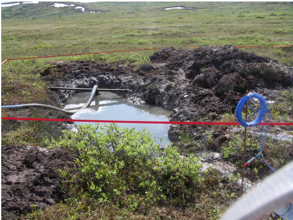
Figure 14. Overflow and recycle sump, drill rig 8413 (No. 4).
