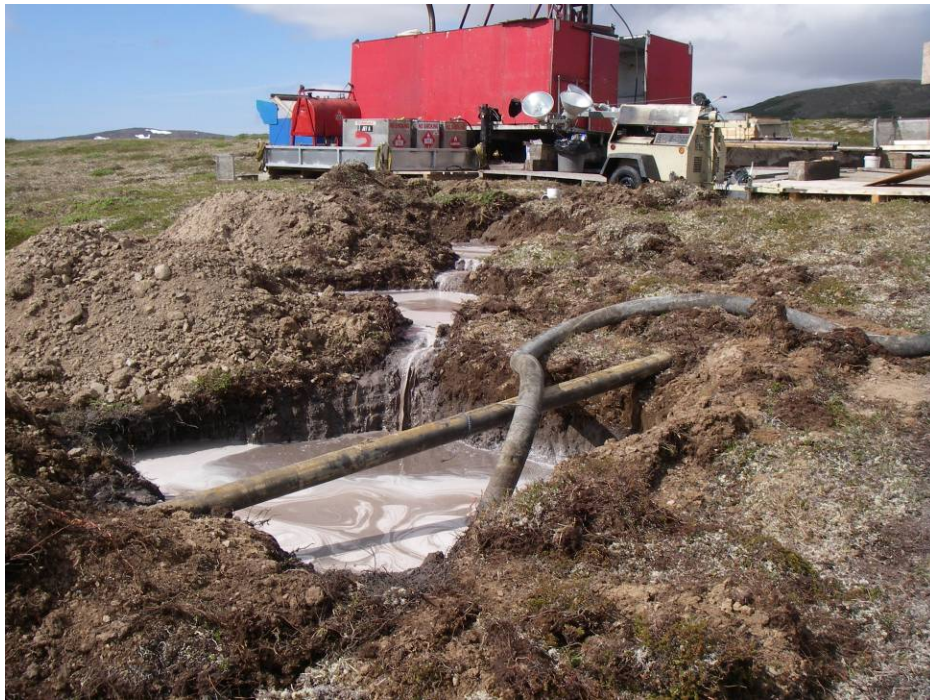
Figure 11. Overflow and recycle water sumps, drill rig 8411 (No. 3).
