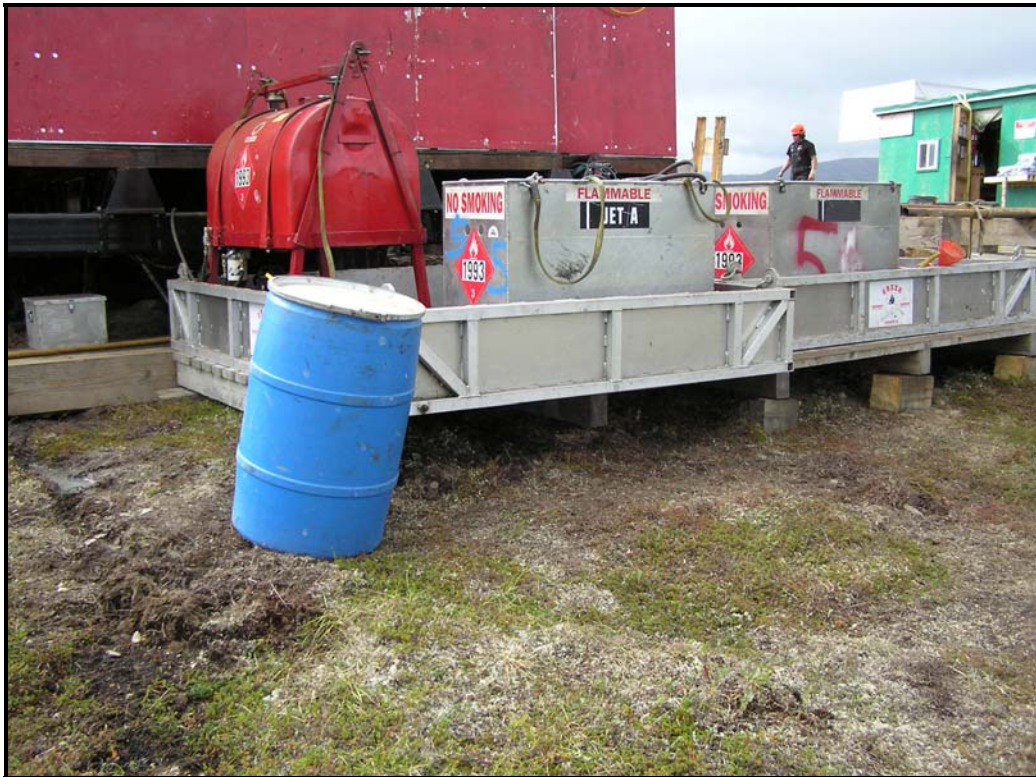
Figure 17: Fuel storage for Rig # 5.
