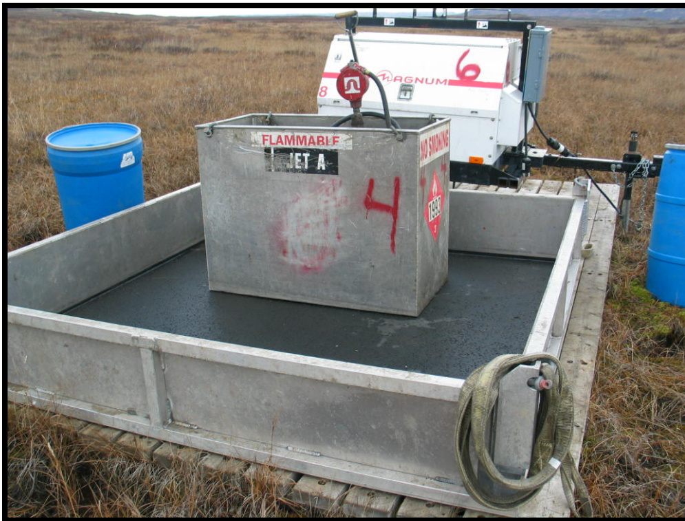
Figure #10: Fuel containment for water pump at Drill #2.
