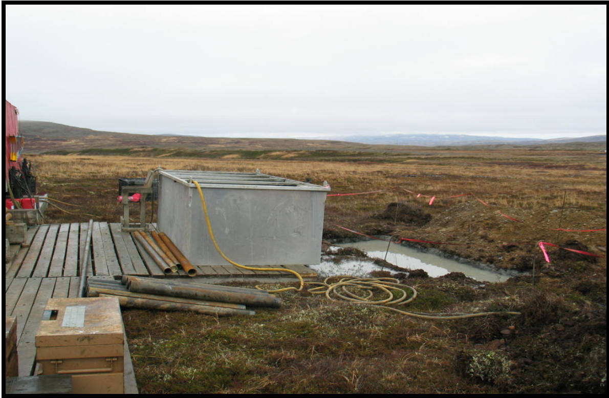
Figure #3: Drill #4. Tank for recycling drilling fluid. Sump is for excess drilling fluid.
