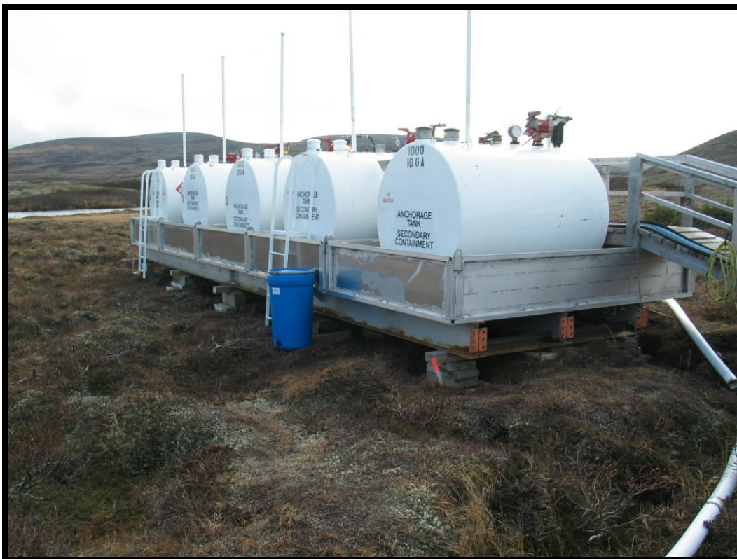
Figure 18: Fuel tanks at Big Wiggly Lake
