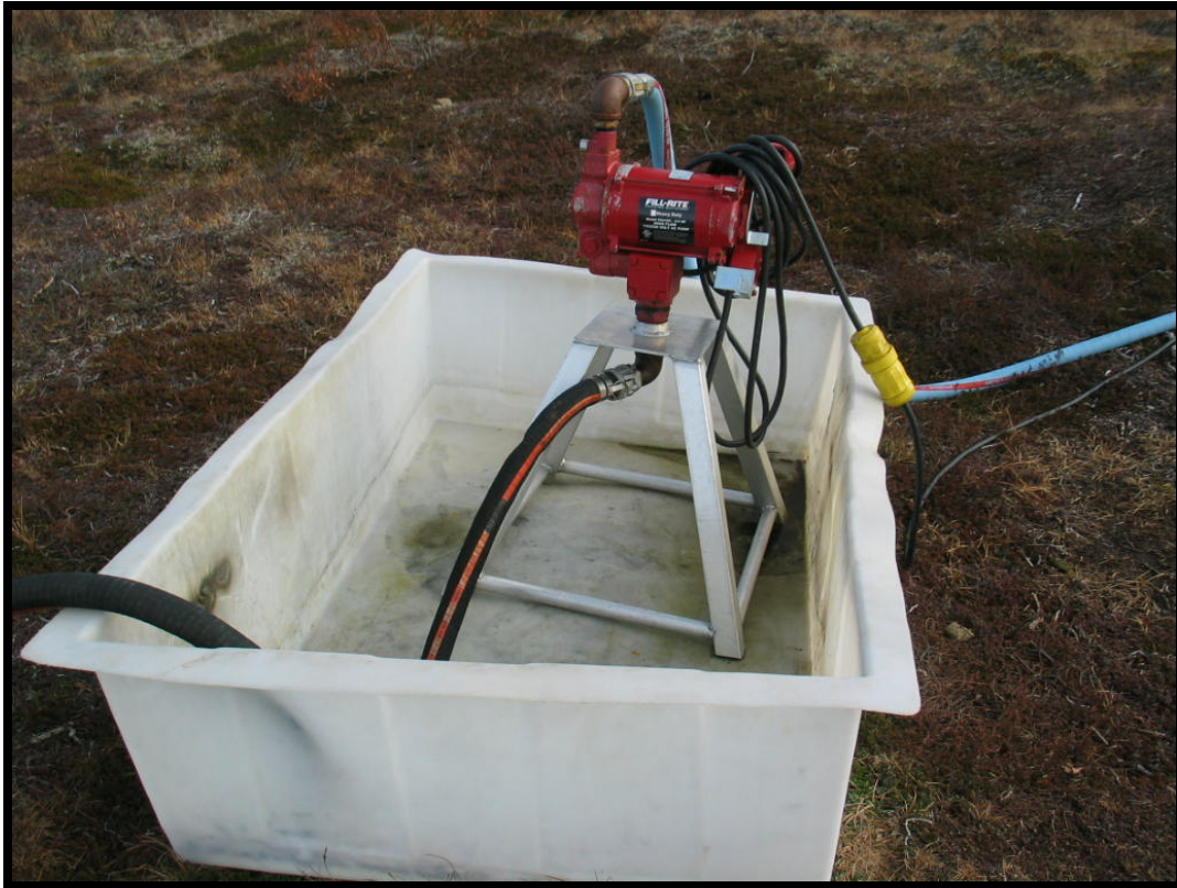
Figure 19: Fuel transfer pump at Big Wiggly
