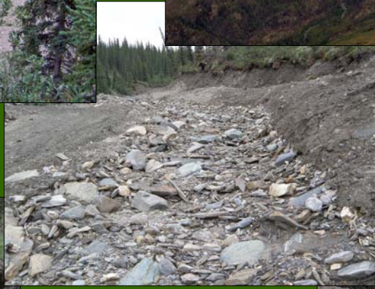
Re-contoured embankments and stable stream channel of placed cobbles and boulders on California Creek
