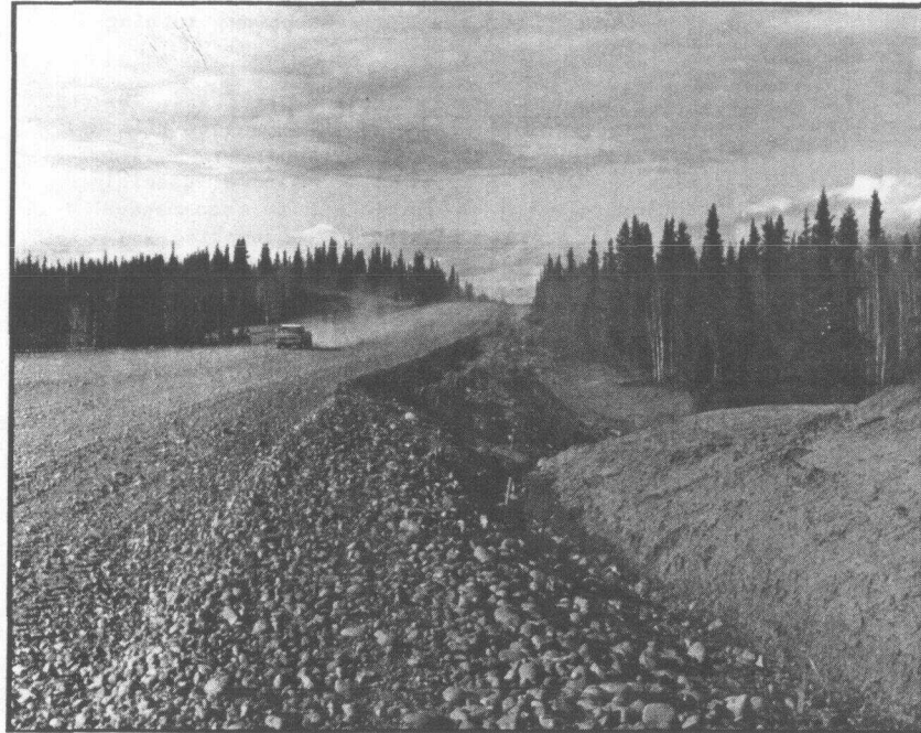
Recent construction and upgrading have left visible scars in the right of way.
